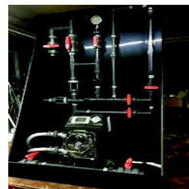
Single Dosing System
